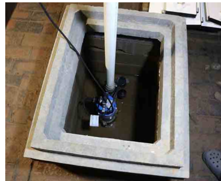
Two more pumps in the cellar.
